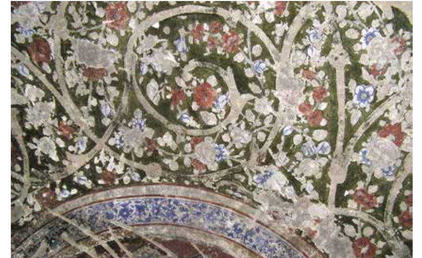
Fig. 103 Wall paintings in the ante- and main room of the bath, detail, 2004
