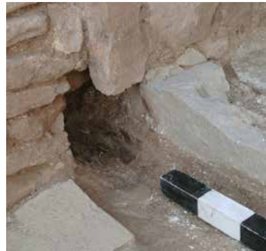
Fig. 393 Central entrance room (Room 1), lateral recesses for square timbers to stabilise the steps
