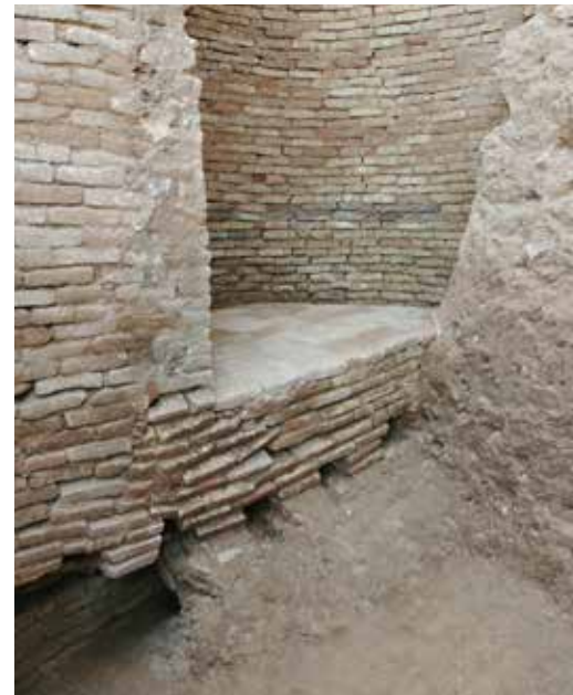
Fig. 388 'Niche Room' (Room 6), recesses in the foundation for the placement of horizontal beams
