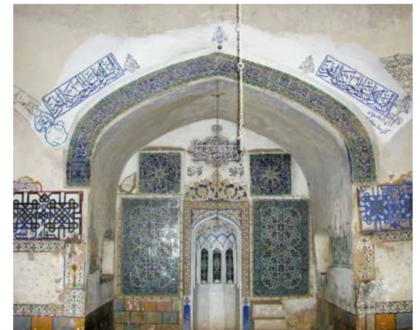
Fig. 909 Western wall with mihrab and super-imposed and renewed decorations from different periods
