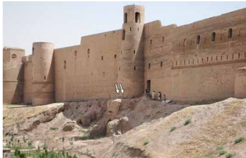
Fig. 560 The gateway area prior to the 2008 excavations, localisation of the cracks in Tower XVIII; from west
