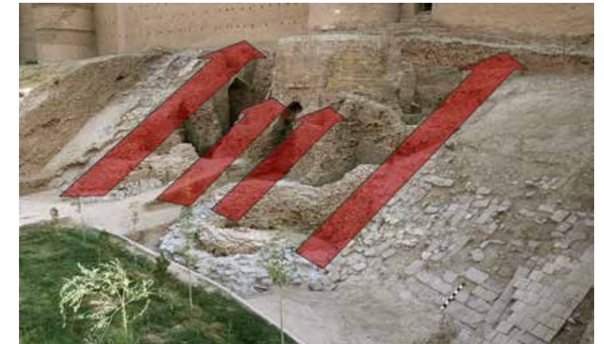
Fig. 562 Gateway at the end of the excavation 2008, schematic display of the necessary supportive system (cp. Fig. 563)
