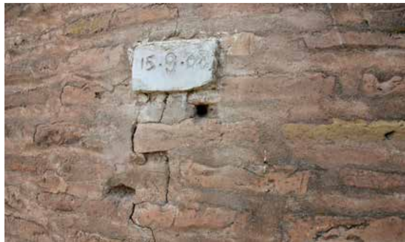
Fig. 561 Tower XVIII, above the gateway, setting cracks and plaster seal of 2008
